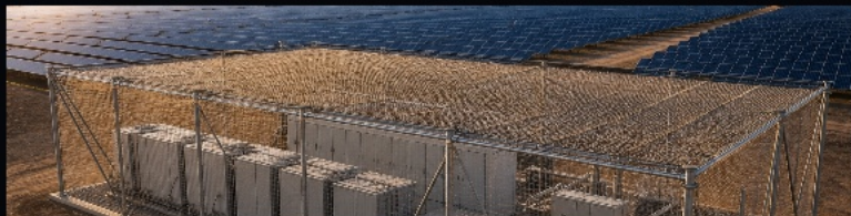
Solar power plants
